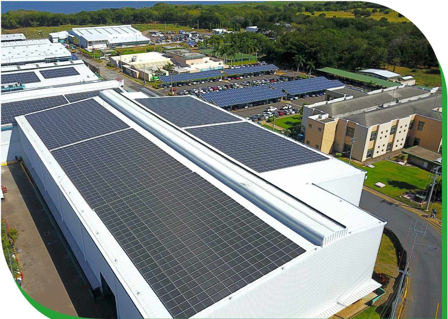
Paneles solares CCN
